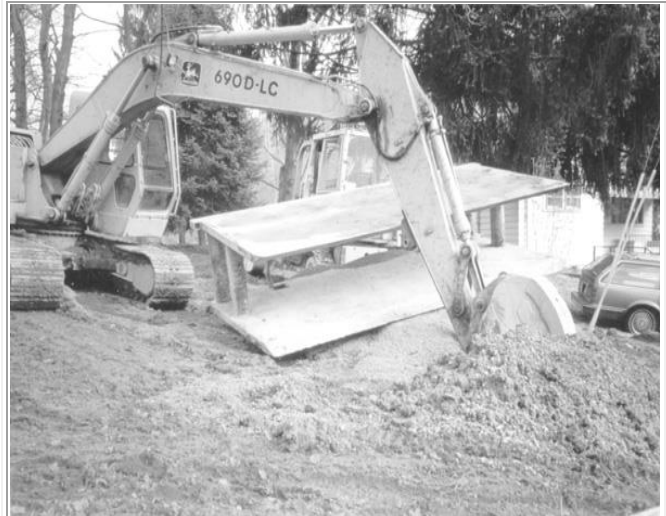
Photo Caption -Safety is of utmost importance when installing or repairing distribution lines. The trench box laying here on its side is about to be placed inside a recently excavated trench. The box shields workers from cave-ins by shoring up exposed soil walls that might fall in otherwise. Photo by Jamie Knotts.
